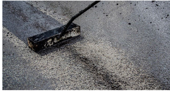
Above | A one pass screed application of TexBand over a large surface crack
