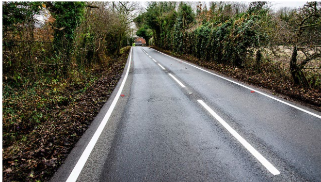
Above | A completed stretch of Cartridge Road with fresh lines, studs and TexBand repairs.
