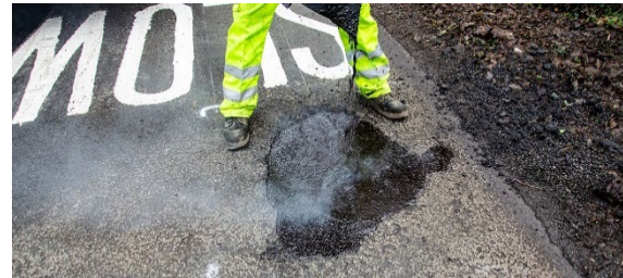
Above | A pothole being filled and left to cure before the final pass
