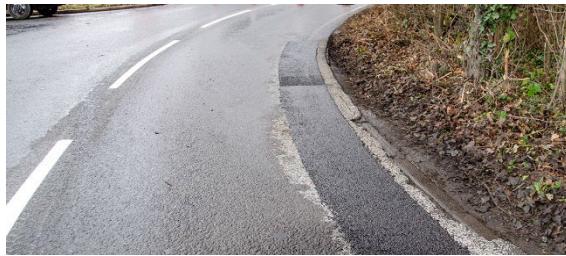
Above | A large surface crack around a bend freshly repaired with TexBand
