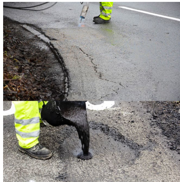
Above | More images of the task in hand to repair surface cracks and large potholes up to 70mm deep and nearly 1m diameter.
